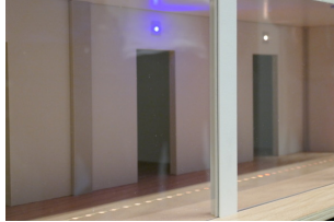
(e) 2022: fire alert and emergency guiding system
